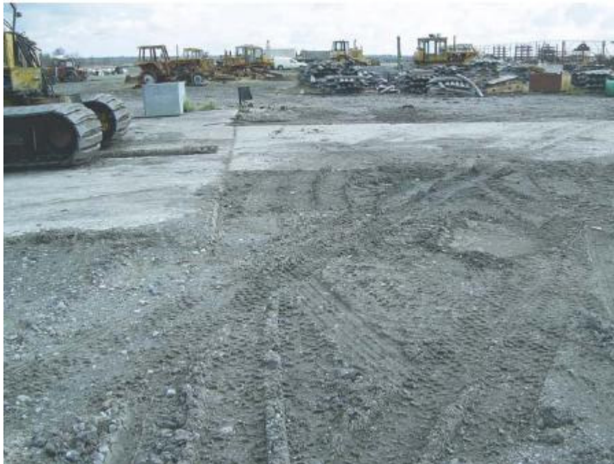
Plate 12.1 Area Immediately to the North of the Current Derrygreenagh Works looking East
